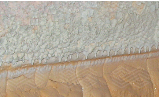
Silica crown is dripping on Superstructure blocks
