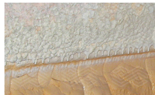
Silica crown is dripping on Superstructure blocks
