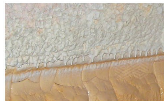
Silica crown is dripping on Superstructure blocks
