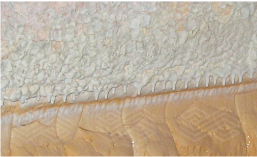
Silica crown is dripping on Superstructure blocks
