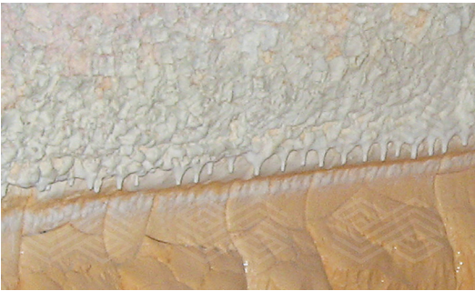
Silica crown is dripping on Superstructure blocks
